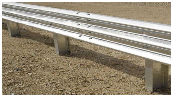
Thrie Beam Guardrail
