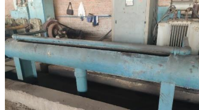
Cooling Part of Tube Mill
