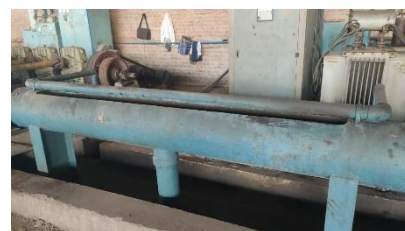
Cooling Part of Tube Mill
