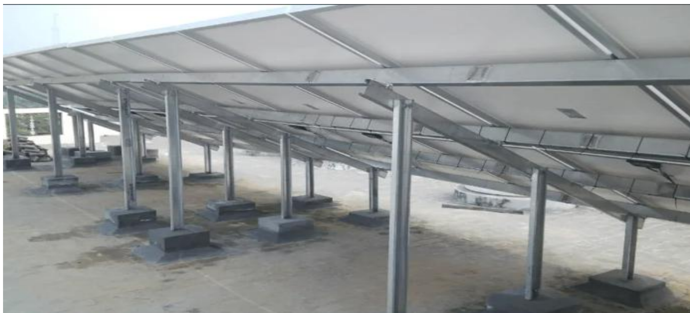
Solar panel mounting structures
